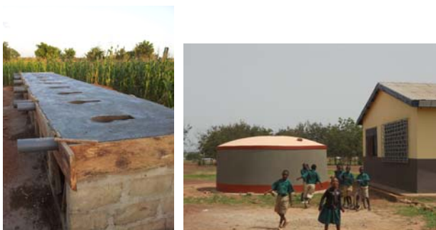
Toilet block under construction in Nyerezee Primary School and a finished tank in Nyankpala School.
