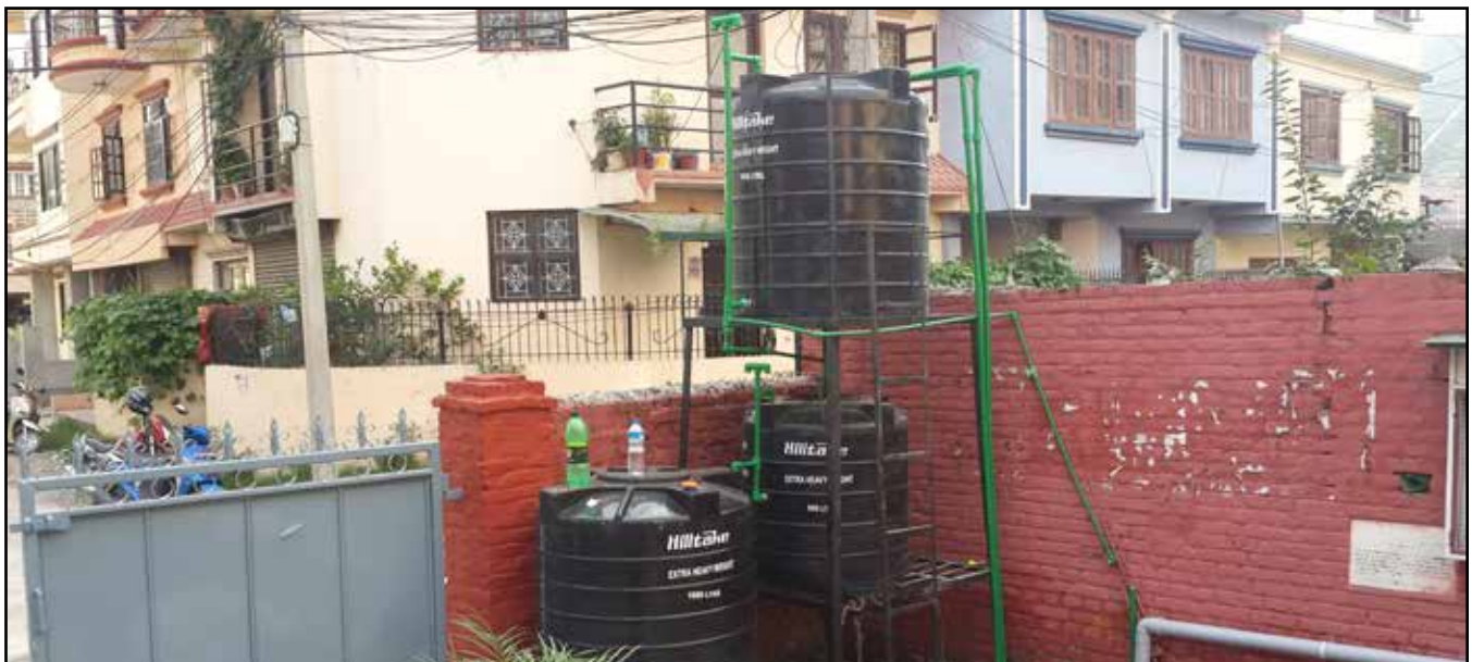
Figure: Rainwater Harvesting System installed at Dallu Awasi, Ward No. 15
