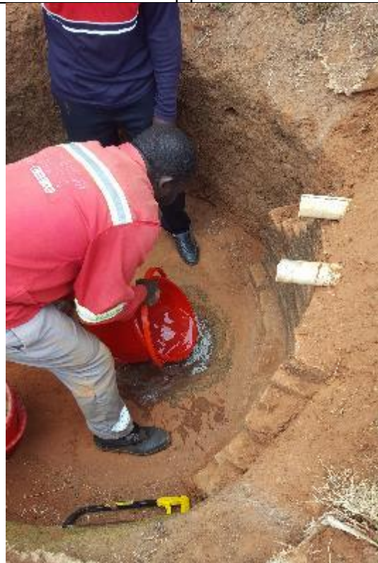
If ready, test the recharge capacity by pouring a few buckets of water
